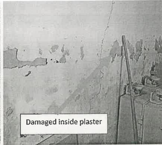
Damaged plaster and mortar situation in wall
