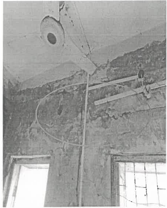
Spalling in ceiling Concrete
