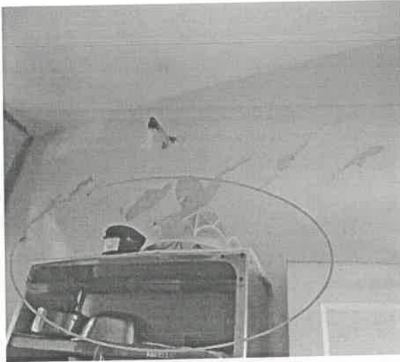
Horizontal cracks in the wall and seepage
