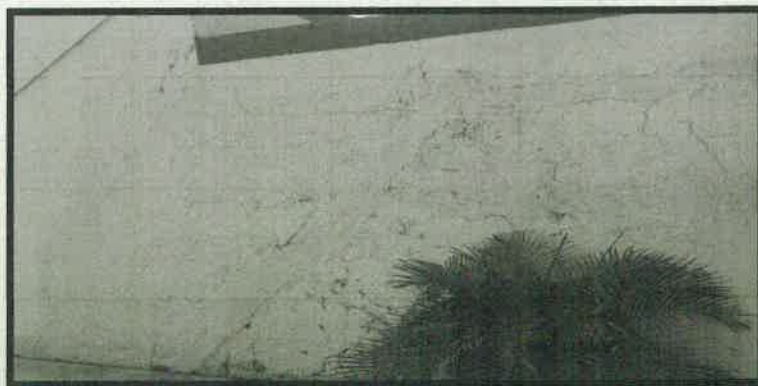
Dampness and cracks in Community Hall building
