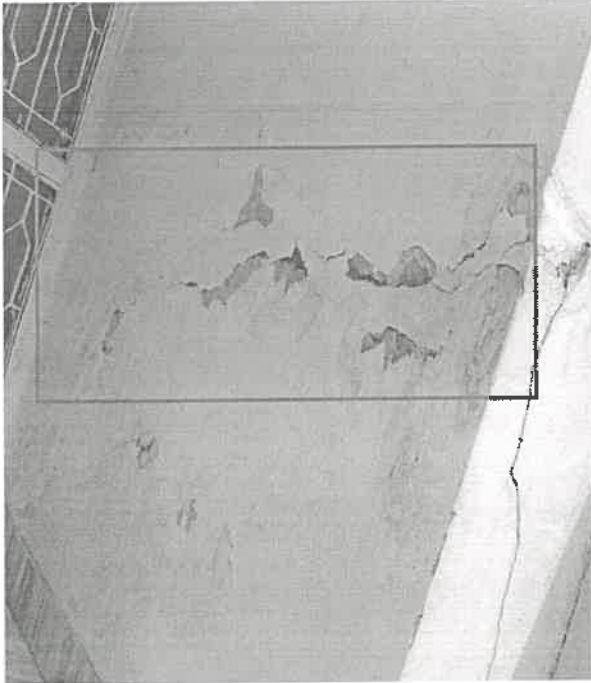
Diagonal cracks in walls
