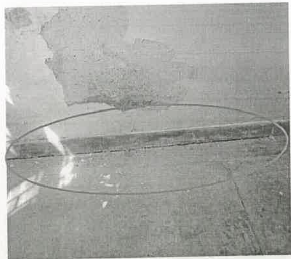
Settling of concrete floor
