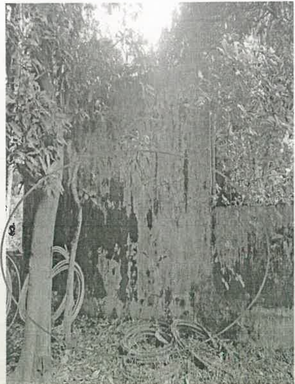
Dampness and vegetation
