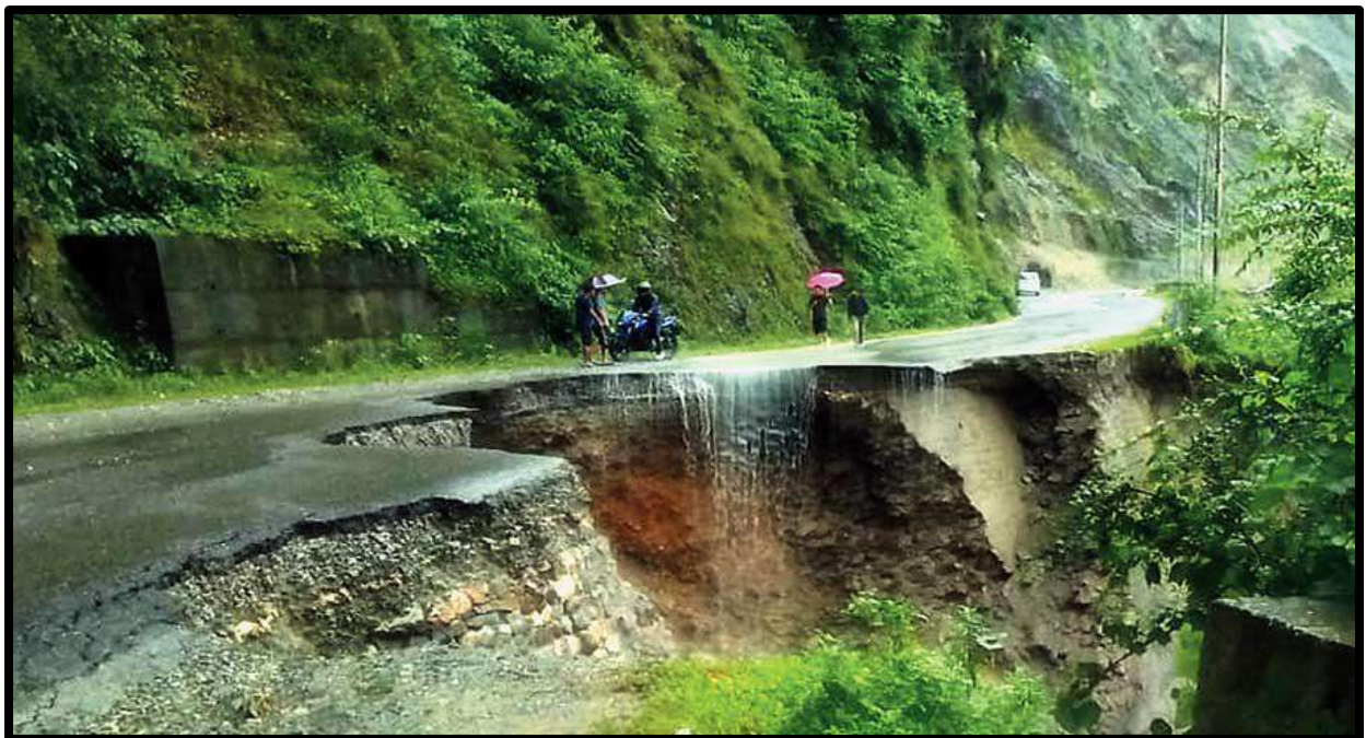
Stretch of NH10 that caved in at Swetijhora
