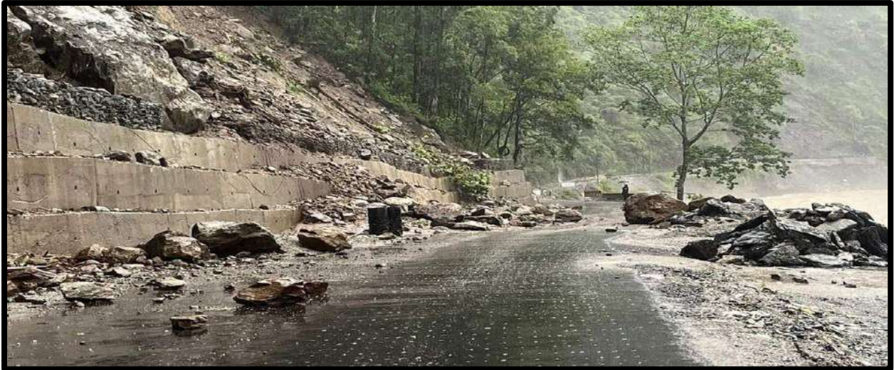
Landslides at Likhubhir
