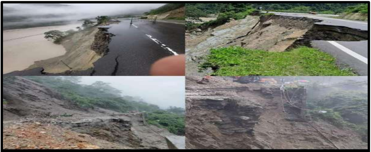
Landslides along NH 10
