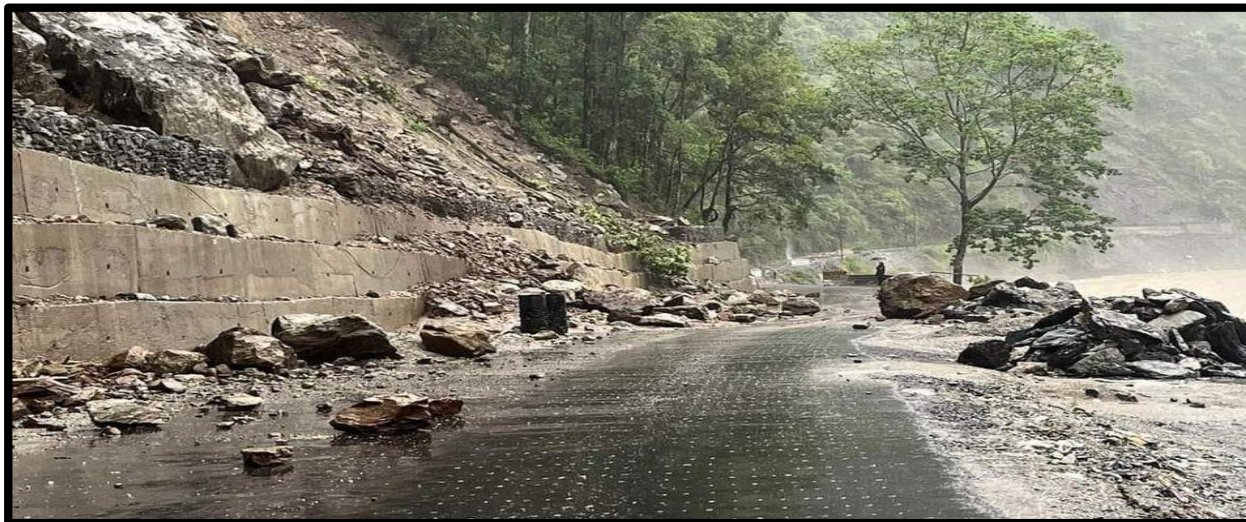
Landslides at Likhubhir
