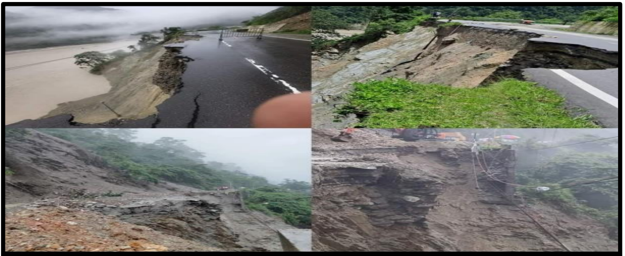
Landslides along NH 10
