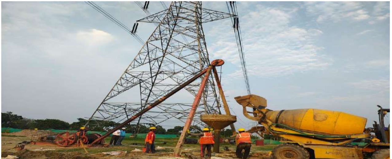
Tower no 439- Bagmati River- Samastipur Bihar
