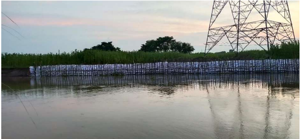
After- Photographs of Tower no. 97 (Tower protection by using Bamboo piling & Geo Bags)
